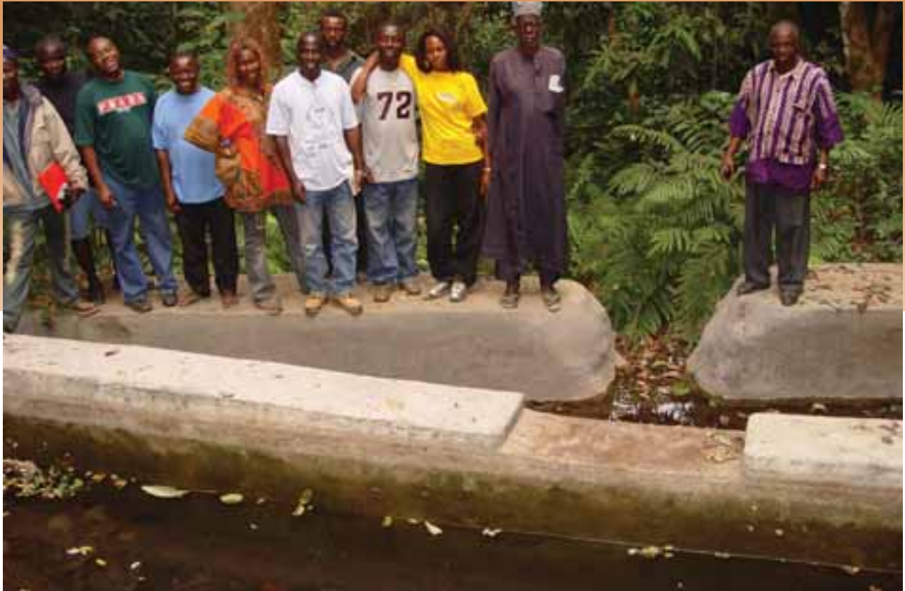
Dam construction for agriculture in a rural area, Sierra Leone. Photo credit: L. Lartigue, USAID.
