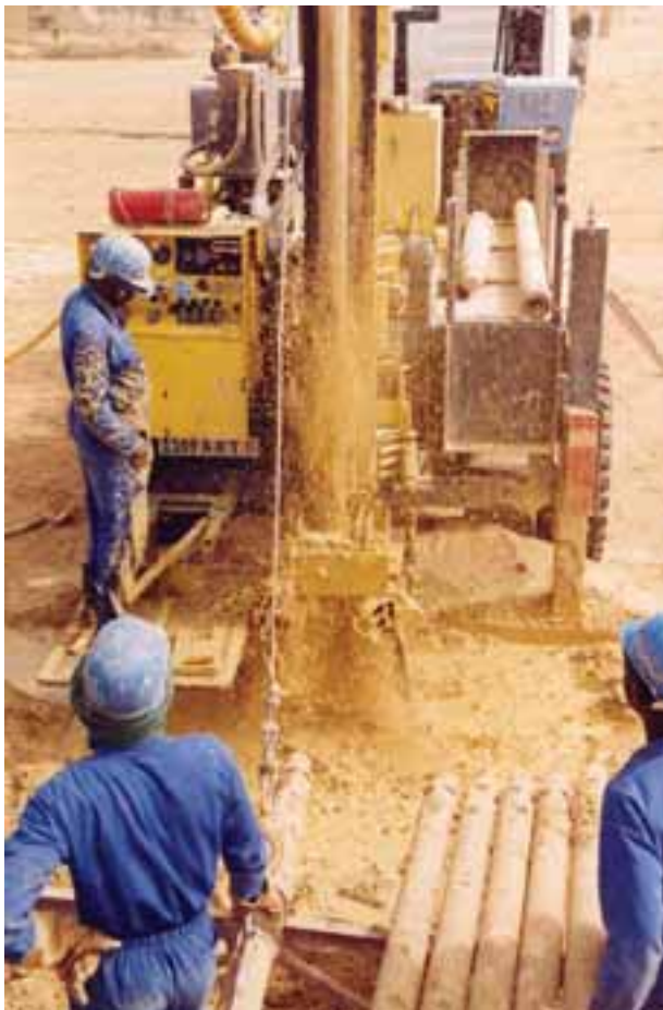
Drilling borehole in the Koro region, Mali. Muddy water spews up from 50 meters beneath the earth's surface. Wells in this region range from 95 to 140 meters deep. Photo credit: USAID.
