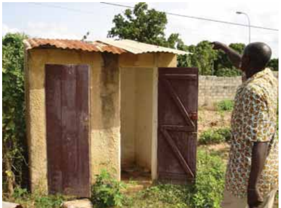
Old latrines, Senegal. Poor hygiene is often cited as a reason parents keep their daughters from going to school. Photo credit: R. Nyberg, USAID.
